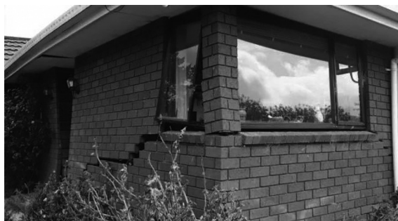
Damage to home in Stillwater, Oklahoma. M 5.6. 3/9/2016. Fuente: Ksn.com
